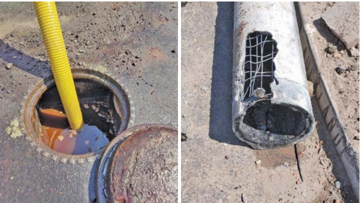
Big fat mess: The sewer pipe in Paarden Eiland (top left), blocked up with fat that had found its way into the sewer system due to some Capetonians' unwise disposal practices. The problem was uncovered shortly after two rising mains had to be replaced in the same street (top right).
